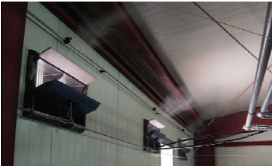
Figure 21: Example Fogging System
